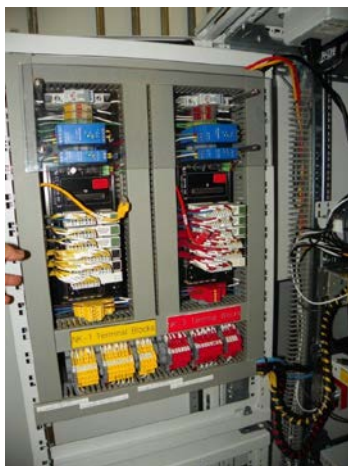
Fig. 12. Cabinet digital I/O system
