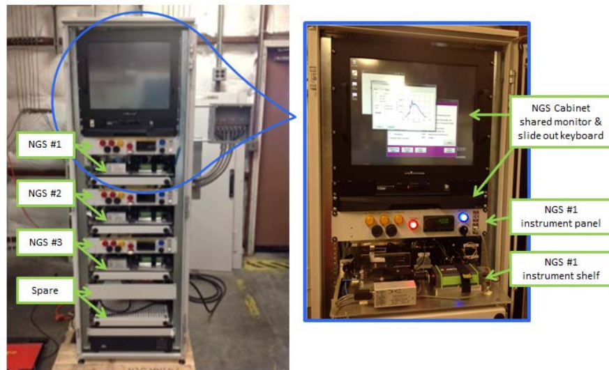
Fig. 9 – HB-Line NGS Cabinet with close up of NGS #1 and shared monitor
